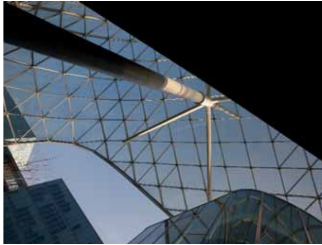
Exhibition center Milan Rho, Italy Structural hollow section to support the "Vela"
